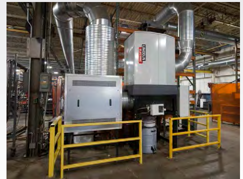
Push/Pull System installed at Elgin Sweeper Company
