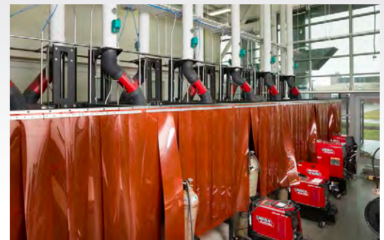
Low Vacuum Central Systems installed at Cuyahoga Community College Welding School
